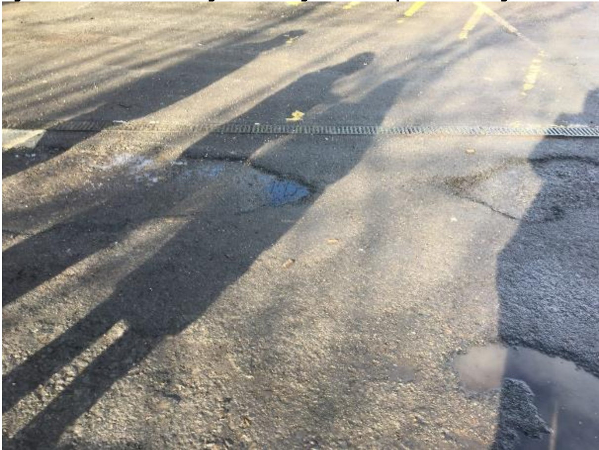
Figure 33: Area within the Designated Parking Area that require Resurfacing
